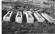
FROM Hikka flush light units are shown under construction in wide area area at March AFB past to test. Lights are located in the end of each concrete "box." Flare units are placed down toward runway ends to provide clearance.
